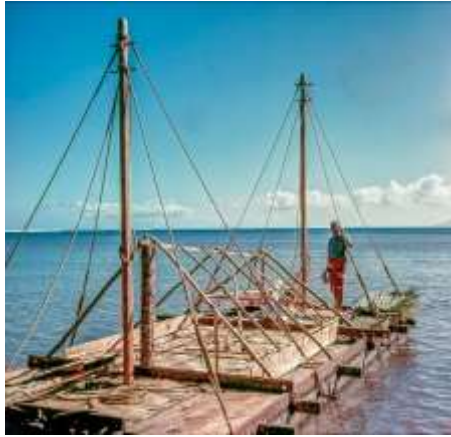
The “Liki Tiki’s” cabin under construction. Everything is lashed together, no metal objects such as bolts, nails, or screws. The ancient Polynesian people did not have metal in any form.
